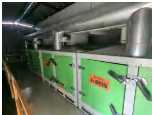
干式过滤+活性炭吸附/脱附+催化燃烧
