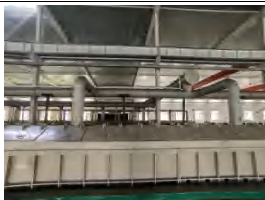
碱洗后水洗槽
