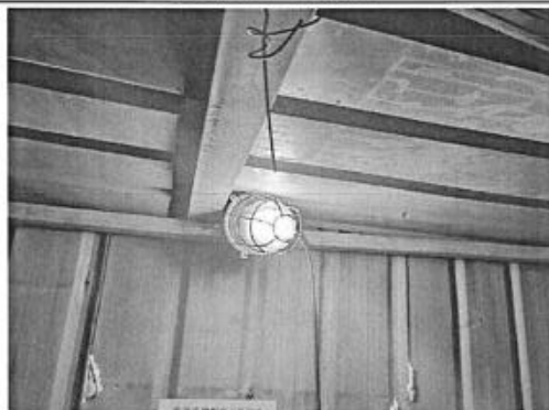
危废间防爆灯
